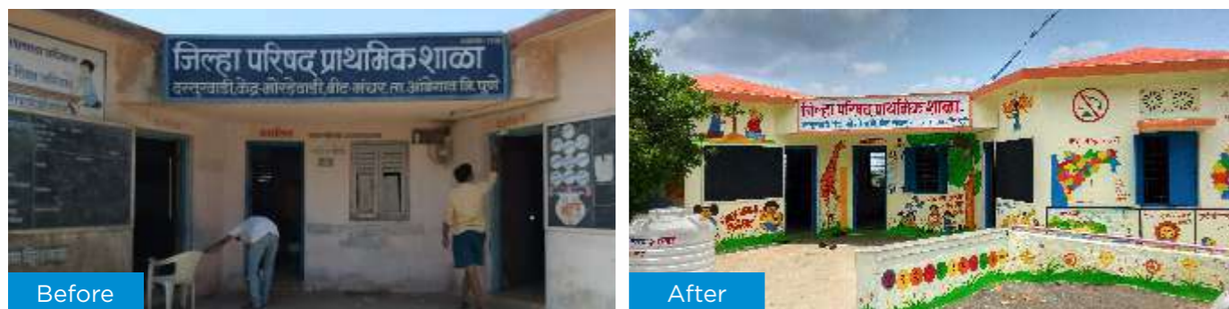
Project: Repairing & painting of Zilla Parishad School Village: Dasturwadi, Tal.: Ambegaon, Dist.: Pune
