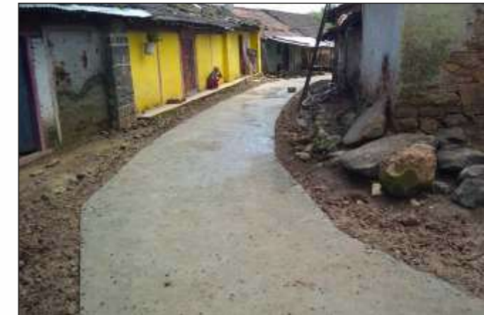
Village: Apti Gangapur (Kh.) Tal.: Amnagaon, Dist.: Pune Construction of internal concrete road
