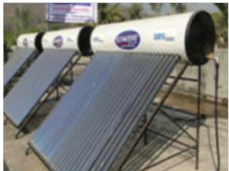
Solar Heater panels installed at SEVADHAM
