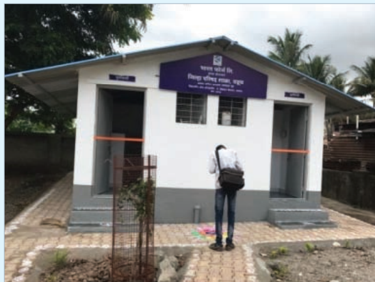
Constructed New Toilets and small internal roads to maintain cleanliness in Zilha Parishad School, Vaduth, Satara.
