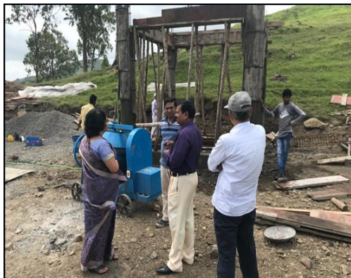
Construction of new water Tank - it is in collaboration with Govt. & BFL.
